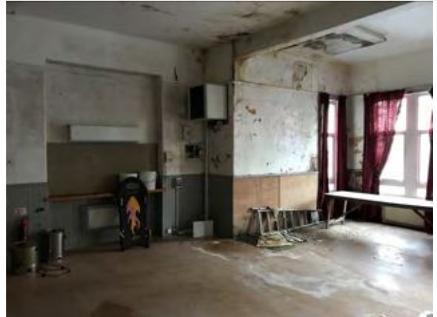
Photo 26. Severe water ingress/damage within room 0/012
