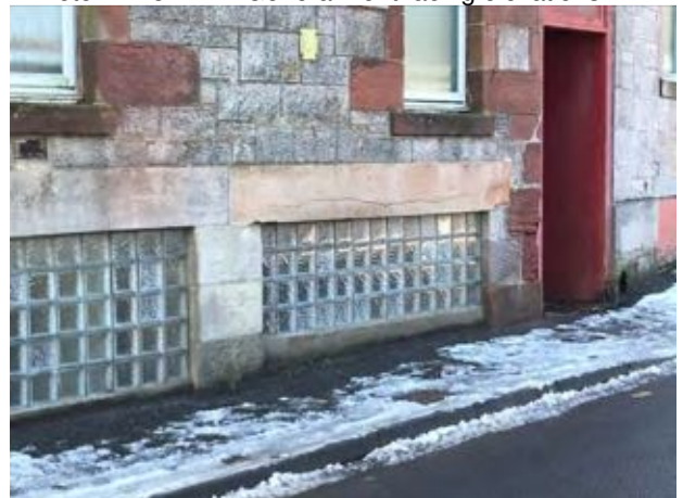
Photo 10. Cracking across lintel to basement windows
