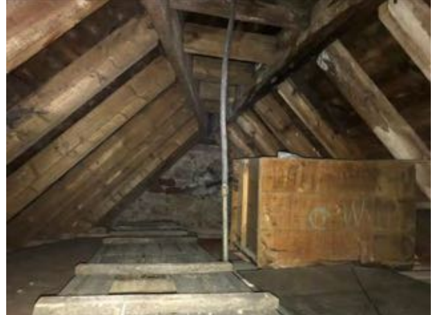
Photo 20. View of water staining and previous timber repairs to roof void
