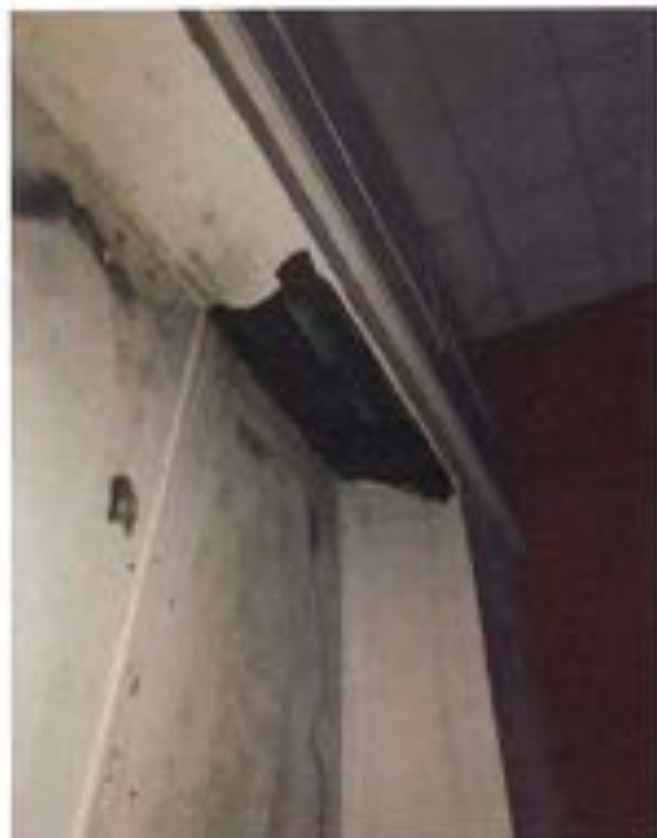
Main hall (Howard Street elevation) - Exposed lintels & water ingress
