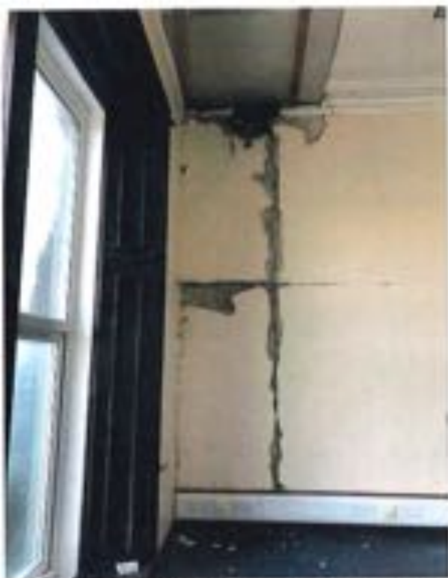
Small hall (along Clifton Street) - Water ingress/dampness
