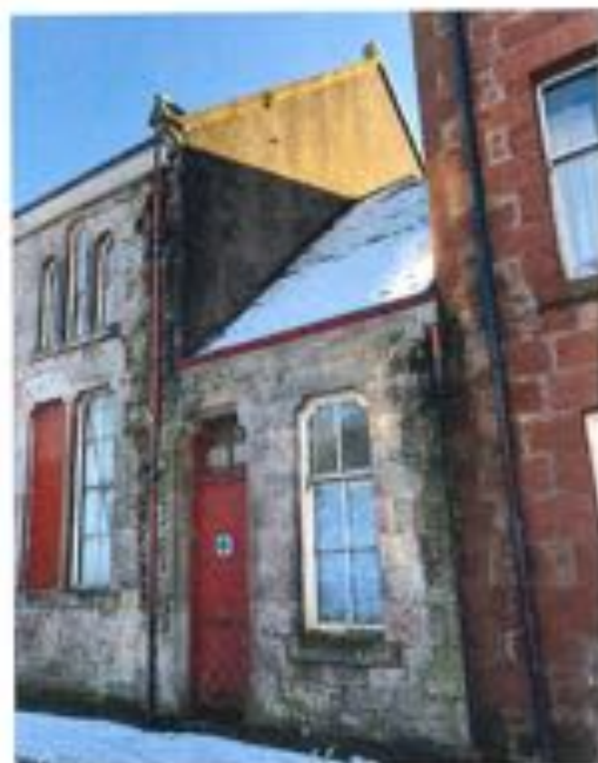
Southwest gable elevation - render cracking
