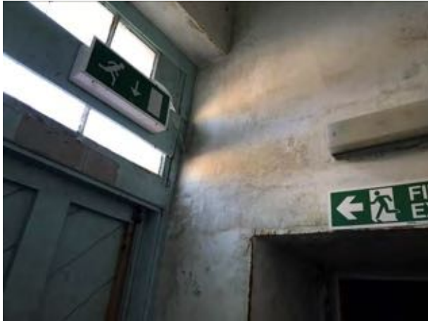
Photo 25. High moisture readings and cracking around door lintels at north-west corner of building
