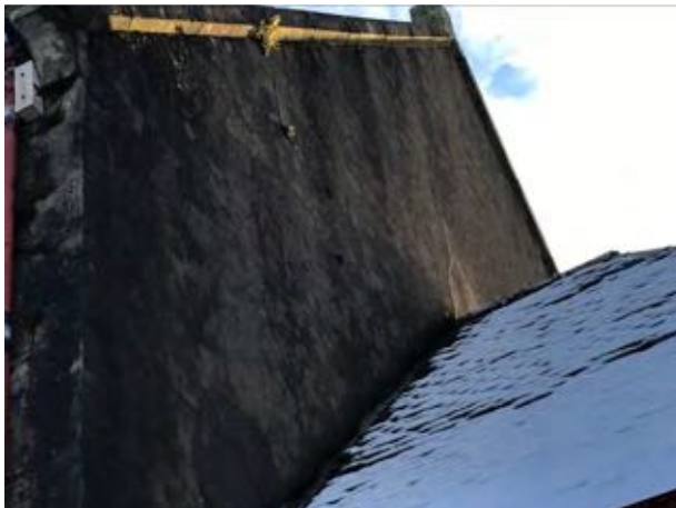
Photo 3. Cracking to high level render
