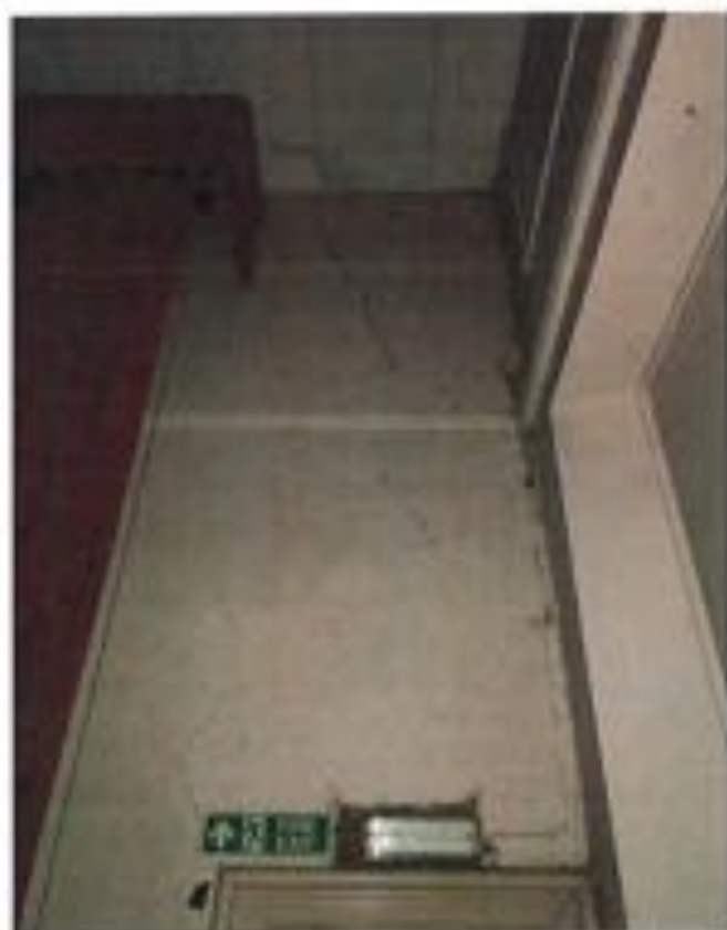
Main hall rear wall (Southwest gable) - cracking
