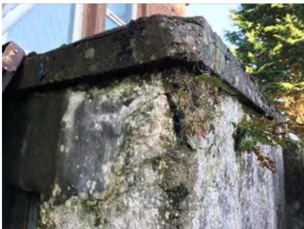
Photo 11. Cracking and vegetation growth to basement toilet entrance
