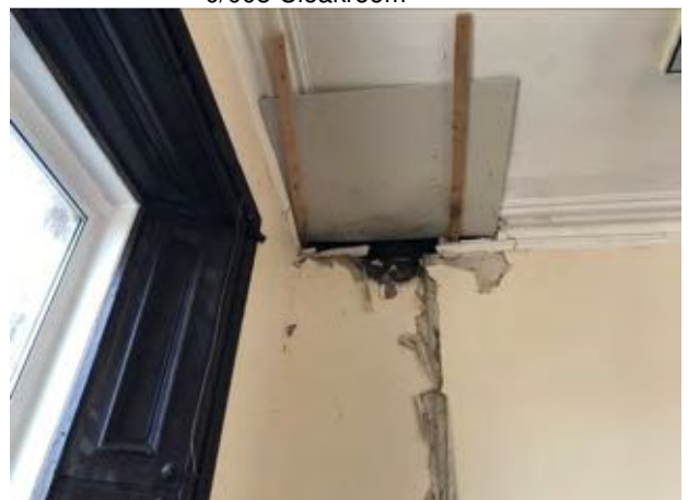
Photo 30. Water damage to ceiling within room 0/007 Office
