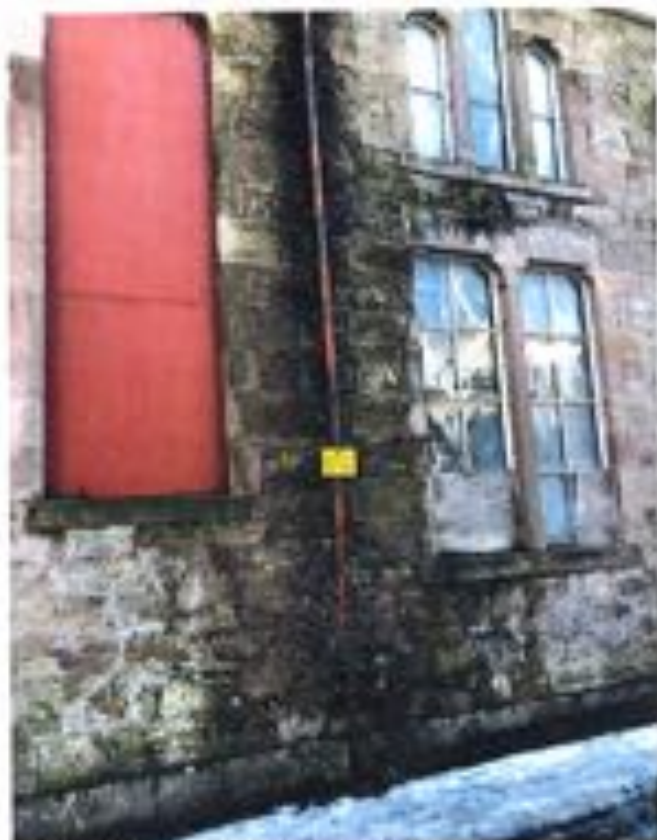
Signs of dampness along Howard Street
