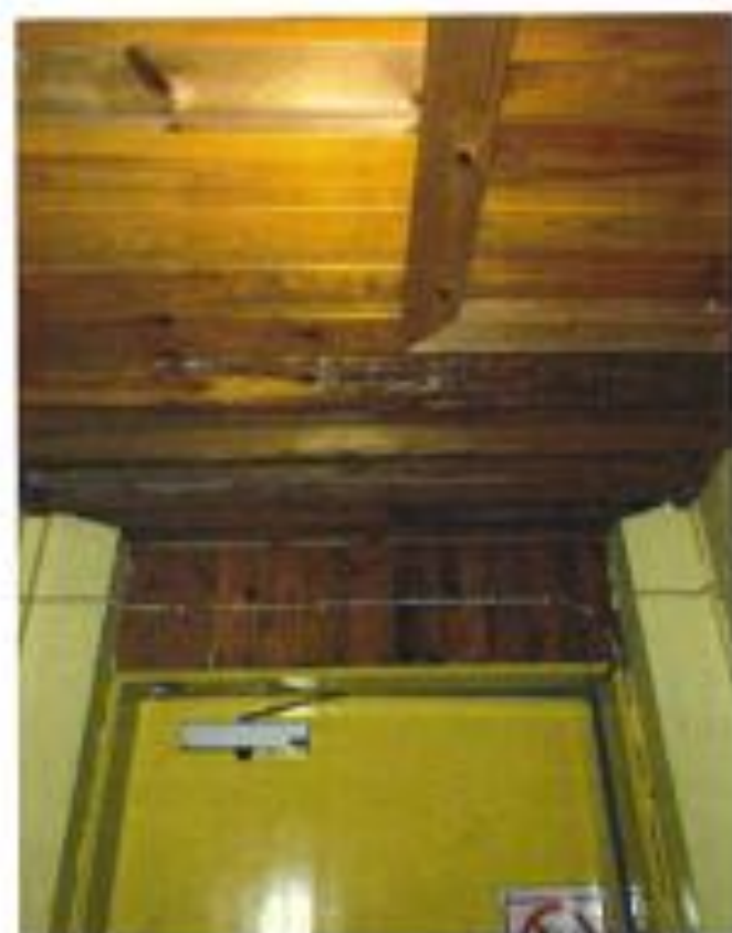
Ground floor hallway - Water ingress/dampness
