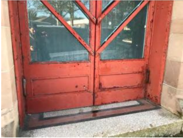
Photo 7. Timber decay to front doors
