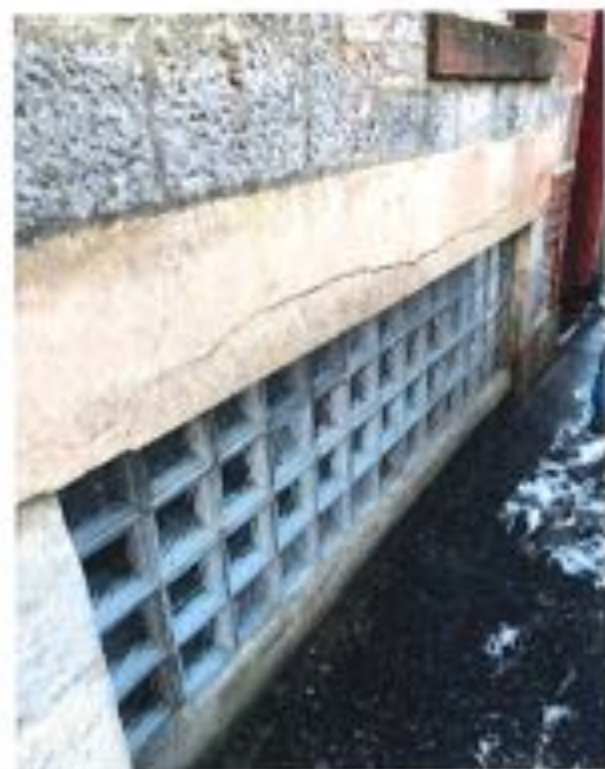
Clifton Street elevation - cracking across lintels
