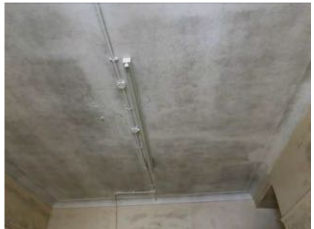
Photo 28. Mould growth to ceiling within room 0/008 Cloakroom
