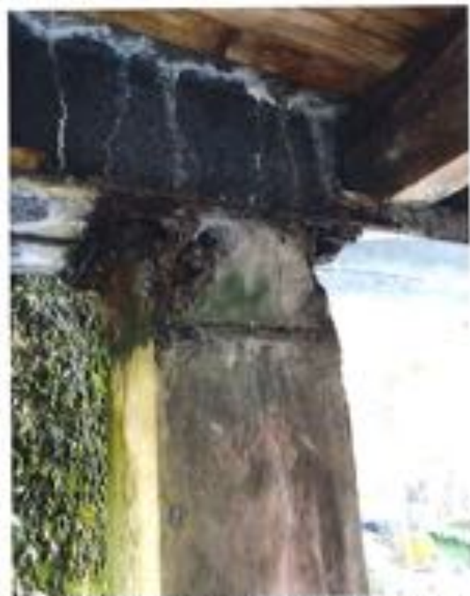
Southeast elevation/undercroft - Damaged steelwork
