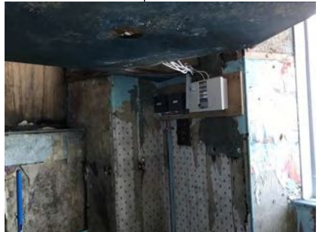
Photo 22. Mould growth and high moisture levels in store at main entrance
