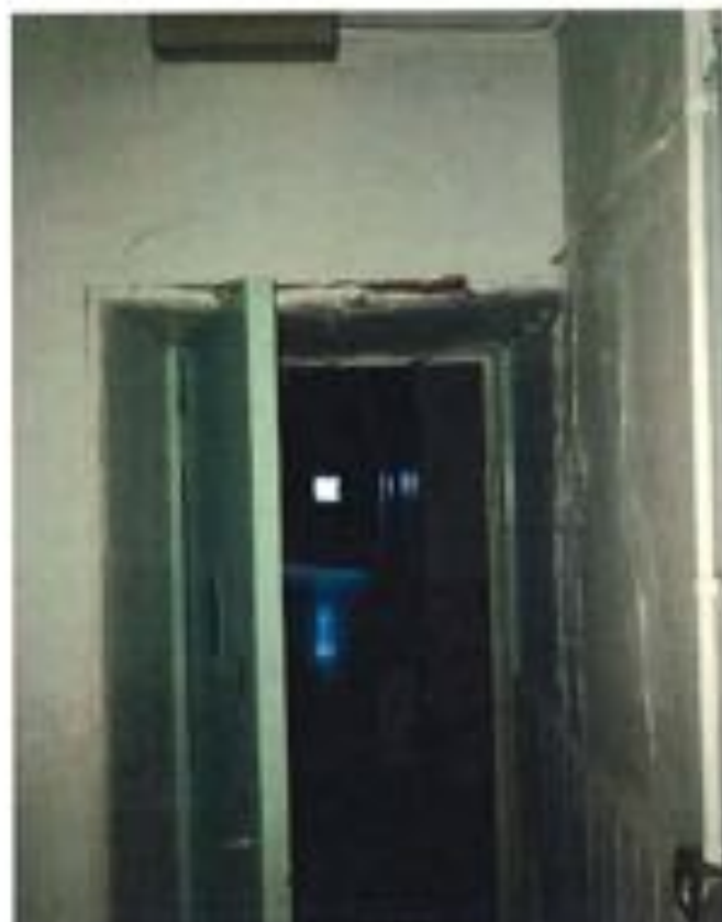
Main hall rear wall (Southwest gable) - damaged lintel(s)
