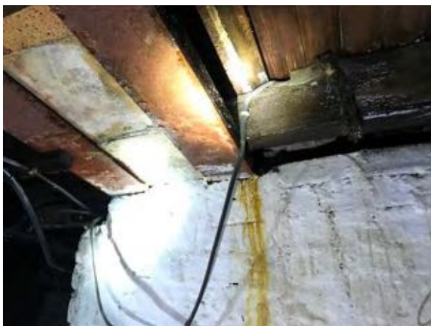
Photo 17. Corrosion to steelwork in basement
