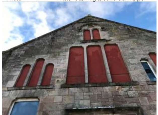
Photo 6. Previous mortar repairs to front elevation
