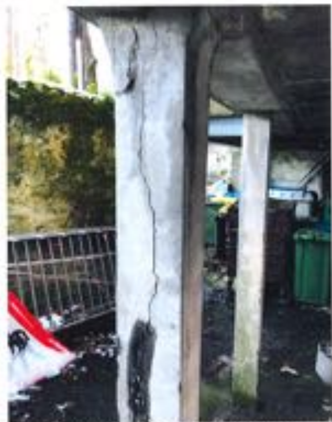
Southeast elevation - Damaged support columns
