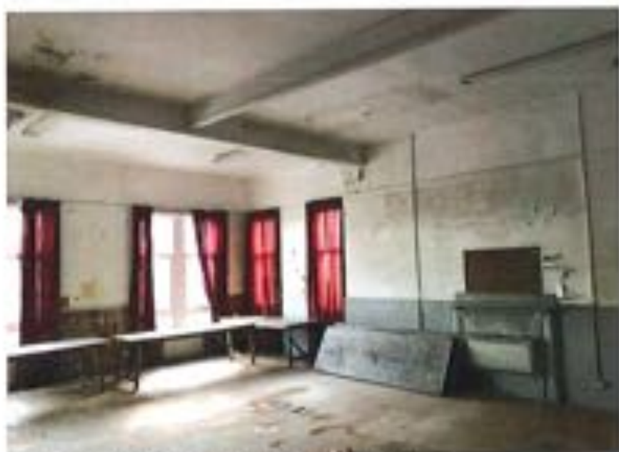
Small rear hall - Water ingress/dampness & damage
