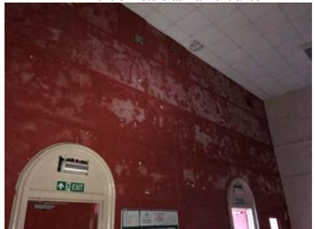
Photo 24. High moisture levels and mould to wall within main hall
