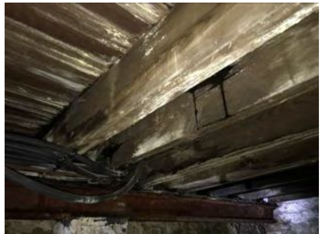
Photo 16. High moisture levels and staining to timbers in basement
