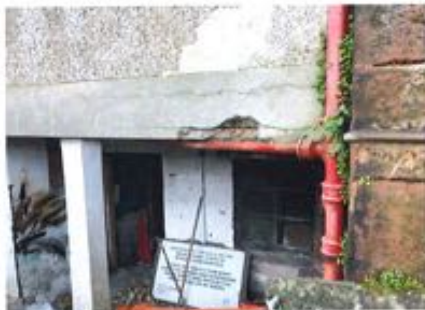
Southeast elevation - Damaged steelwork, concrete & masonry
