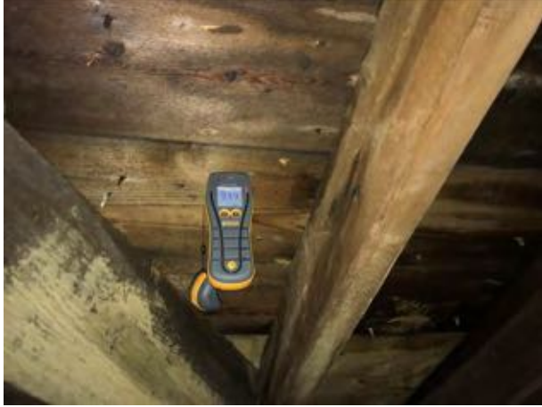
Photo 19. High moisture readings to timber sarking and corroding nail fixings
