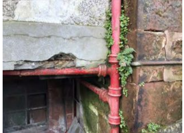
Photo 14. Corrosion to embedded steelwork
