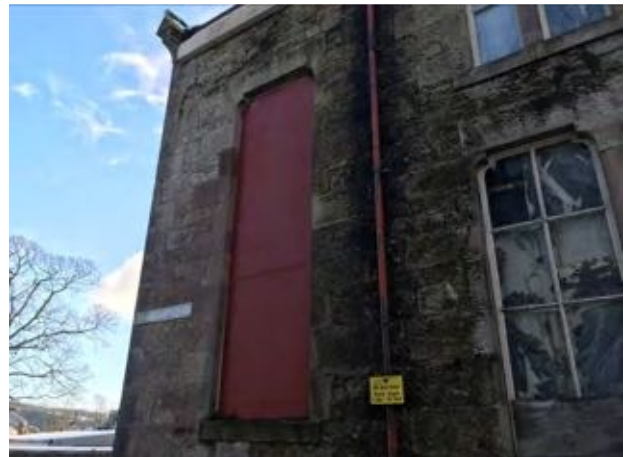
Photo 4. Water staining around downpipe
