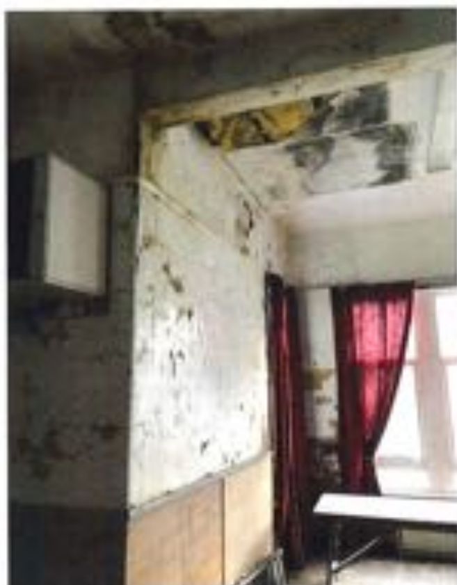
Small rear hall - Water ingress/dampness & damage
