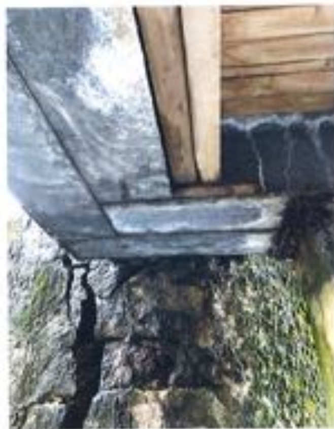
Southeast elevation/undercroft - Damaged masonry
