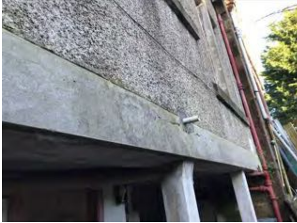
Photo 13. General cracking to structure of south-east extensions
