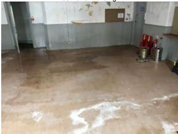
Photo 27. Severe water ingress/damage within room 0/012
