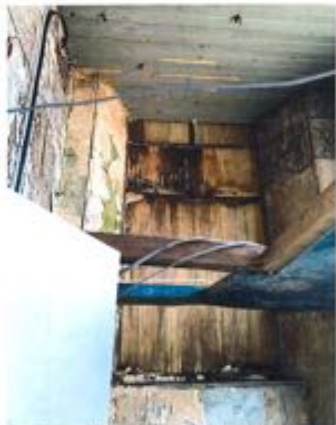
Main hall (Howard Street elevation) - Water ingress/dampness
