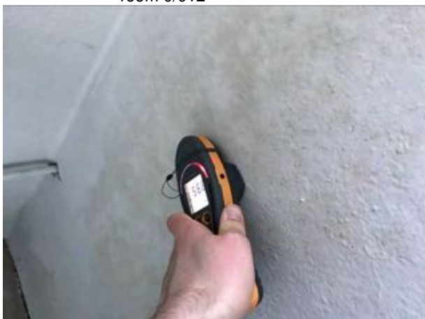
Photo 29. High moisture readings in Male Toilet
