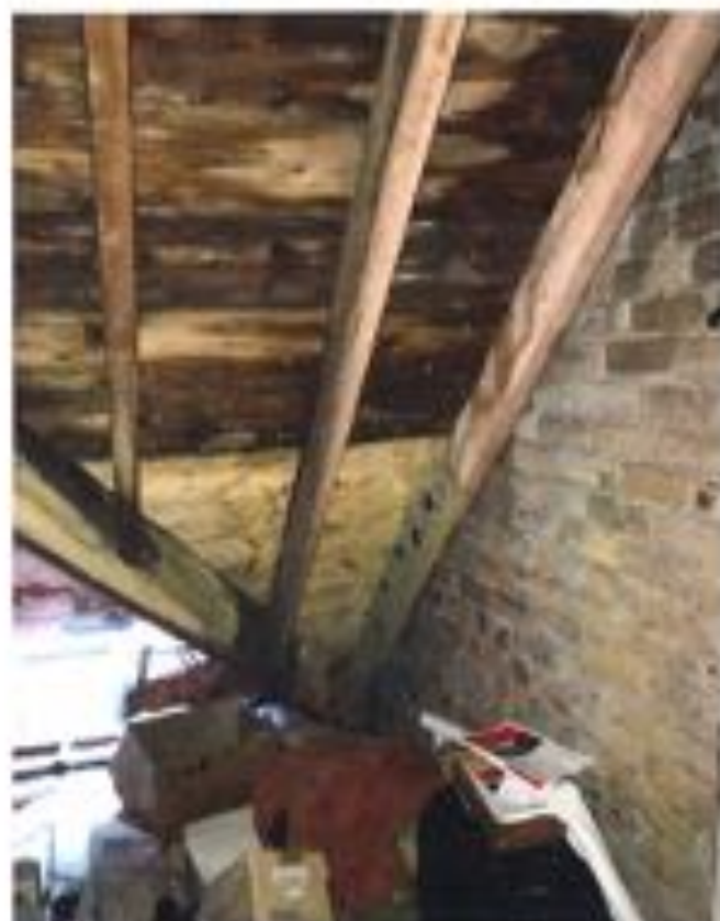
Attic roof void - Signs of dampness/water ingress & previous repairs
